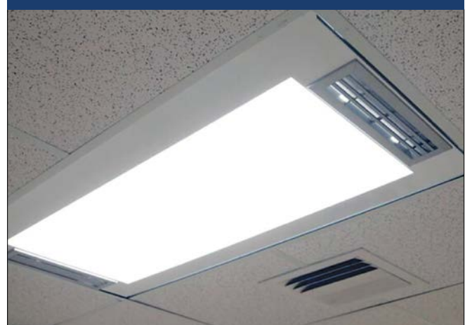
FIGURE 2. UV-C unit installed
